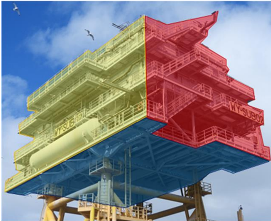
Figure 2b. Image of WOW02 OSS exemplifying how the substation was divided into sides according to aspect and the underside: southside (yellow), eastside (red) and underside (blue).
