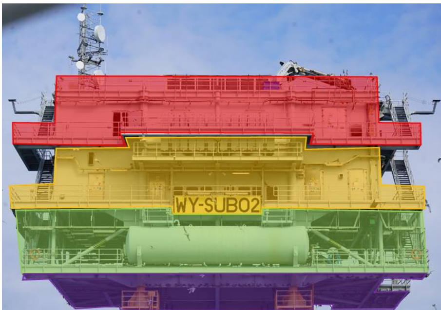
Figure 2c. Image of WOW02 OSS southside exemplifying how the substation was divided into layers: top (red), middle (yellow) and bottom (green) layers. The underside (purple) was categorised as a side.
